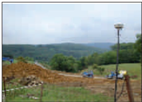
La station satellite est installée
